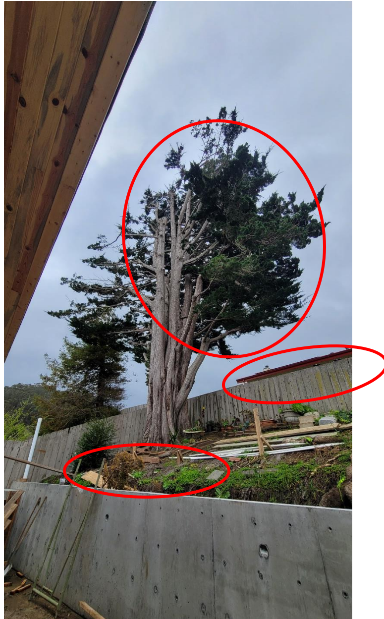
Compromised structural root plate. Unbalanced weighted crown. Neighbor's house
