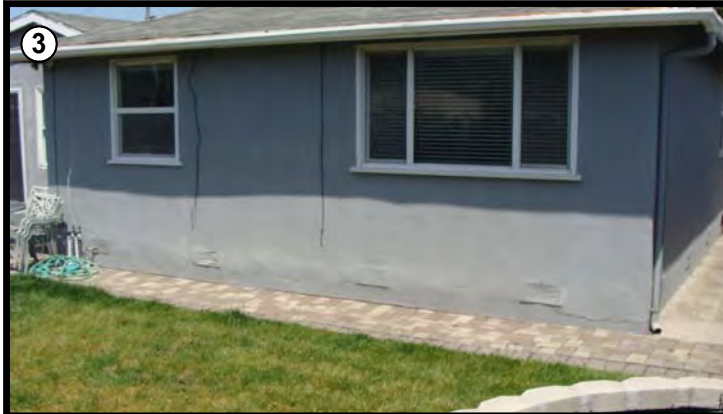
③ View of typical residential house located northwest of the project site. Recently painted with possible patched cracks along base of house.
