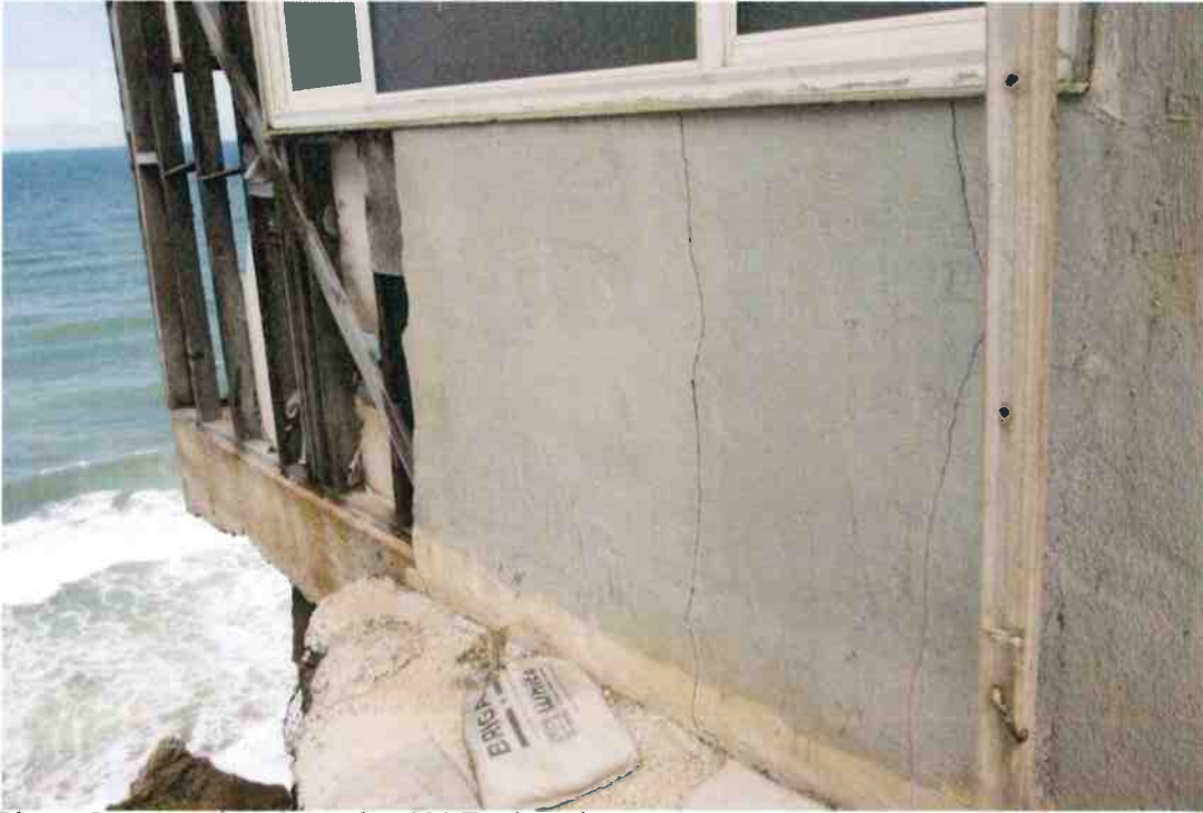
Photo 5B – Tensional Cracks, 320 Esplanade
