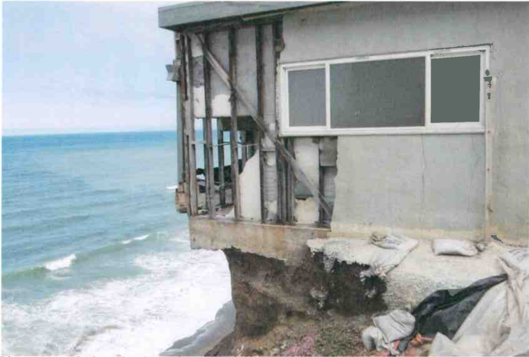
Photo 5A – Undermined Portion of Building, 320 Esplanade
