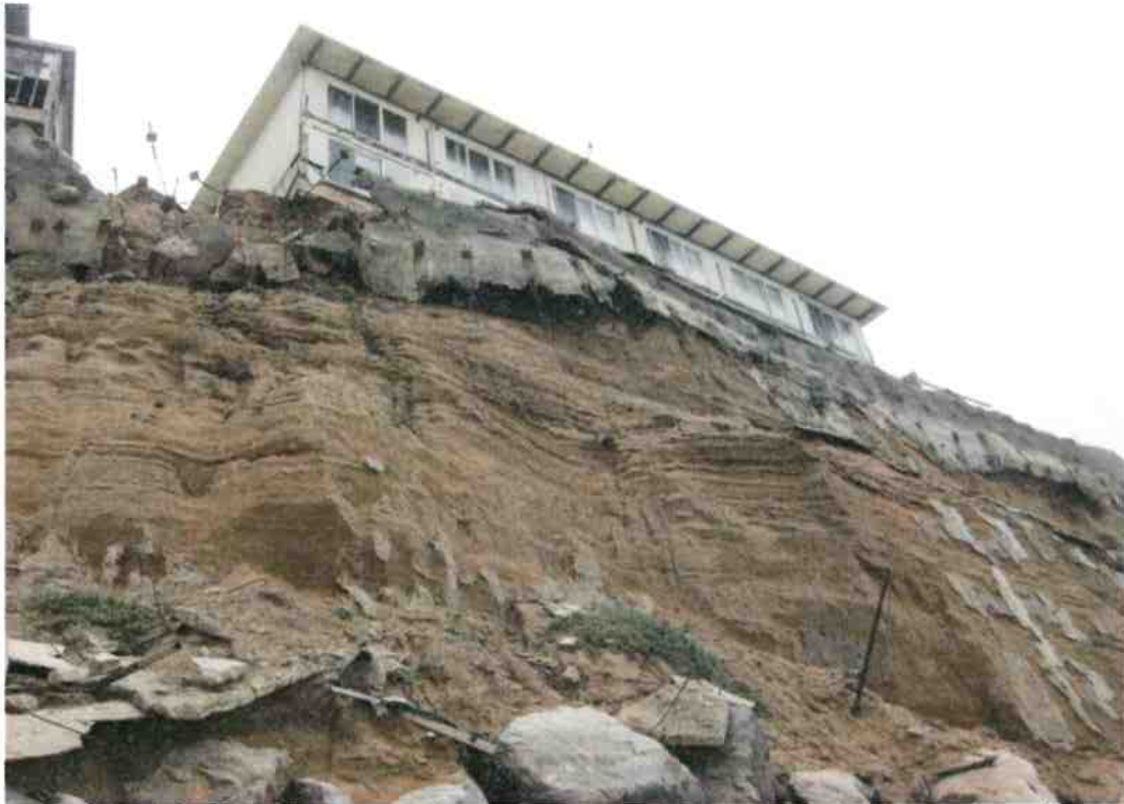
Photo 2B – Debris from Damaged Shotcrete Facing in Foreground, 330 Esplanade
