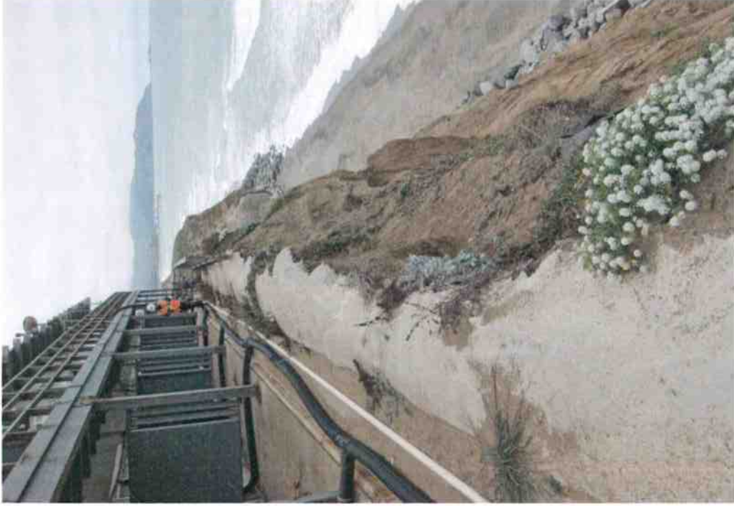
Photo 6A – Building Proximity to Bluff, 320 Esplanade
