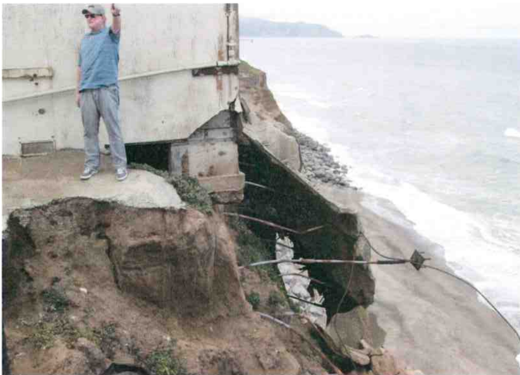
Photo 3B – Northwest Building Corner, Undermined Footing and Shotcrete
