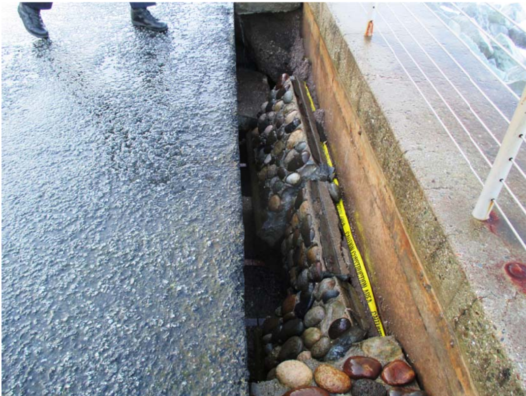
Sink hole at Beach Boulevard promenade near the Paloma Avenue intersection, view facing south
