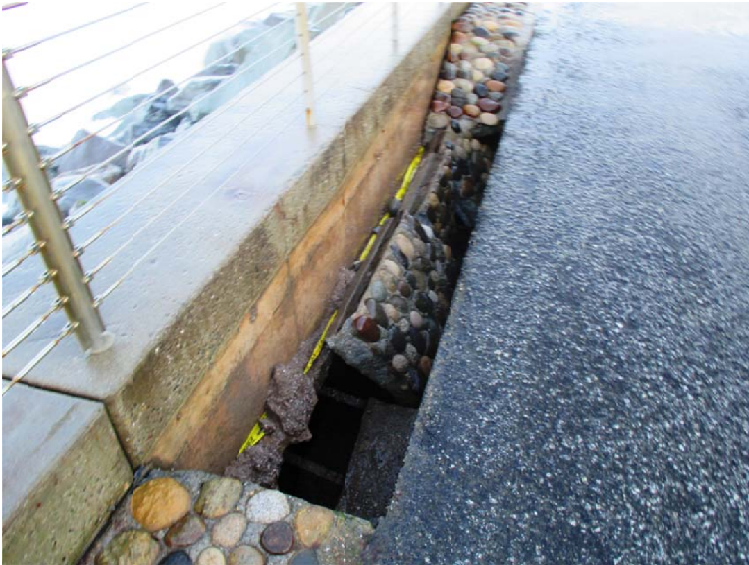
Sink hole at Beach Boulevard promenade near the Paloma Avenue intersection, view facing north
