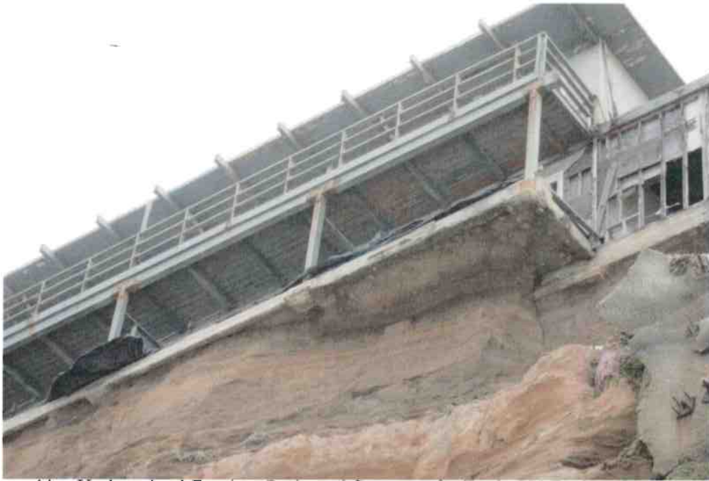
Photo 4A – Undermined Footing, Patio and Supports for Deck, 320 Esplanade
