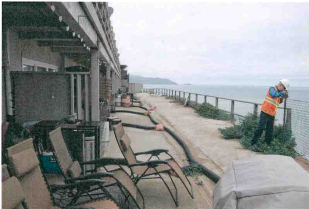
Photo 7B – Comparatively Wide Top of Bluff Area, 310 Esplanade
