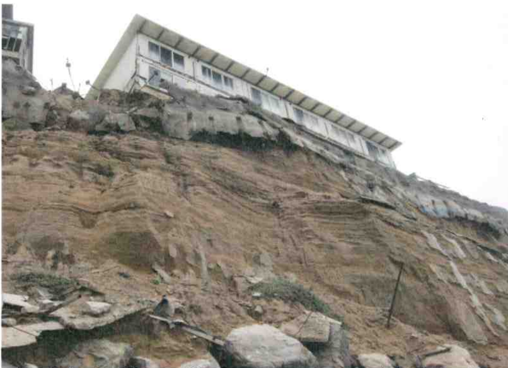
Photo 2B – Debris from Damaged Shotcrete Facing in Foreground, 330 Esplanade
