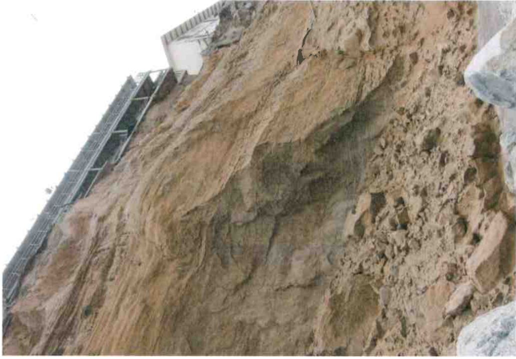
Photo 6b – Recent Cavity Failure, 320 Esplanade
