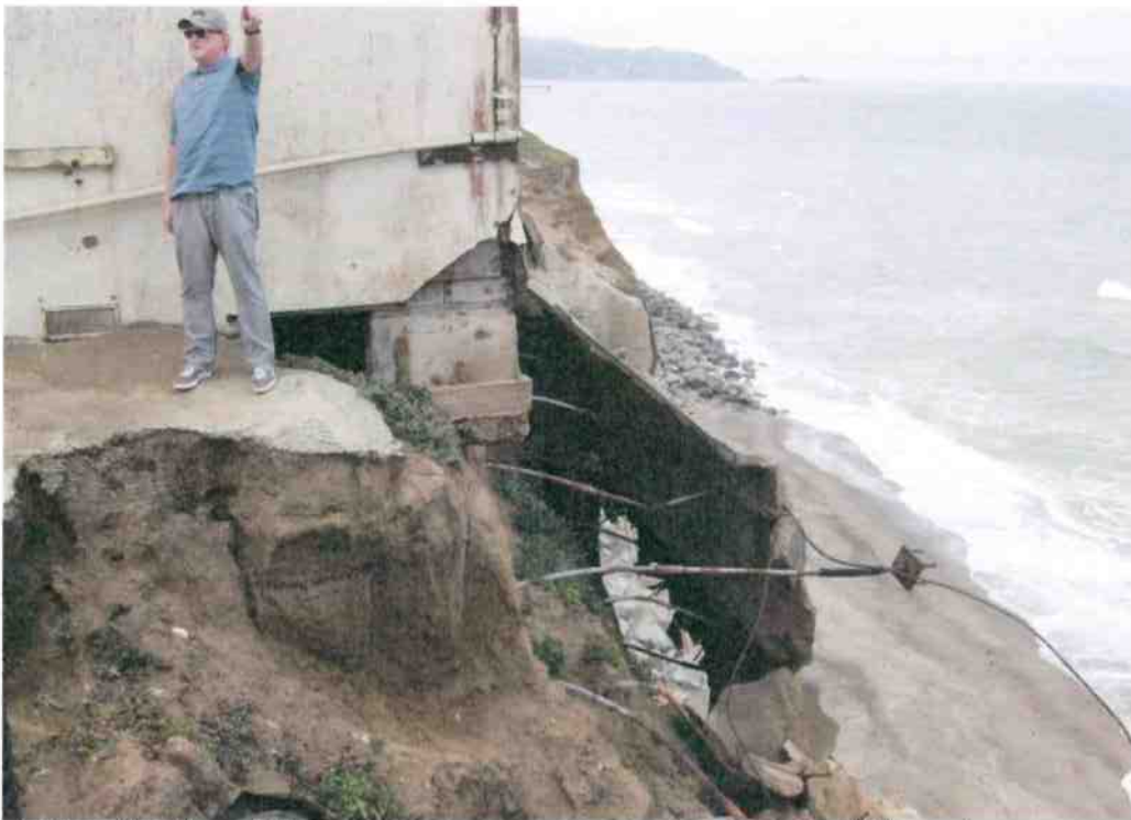
Photo 3B – Northwest Building Corner, Undermined Footing and Shotcrete
