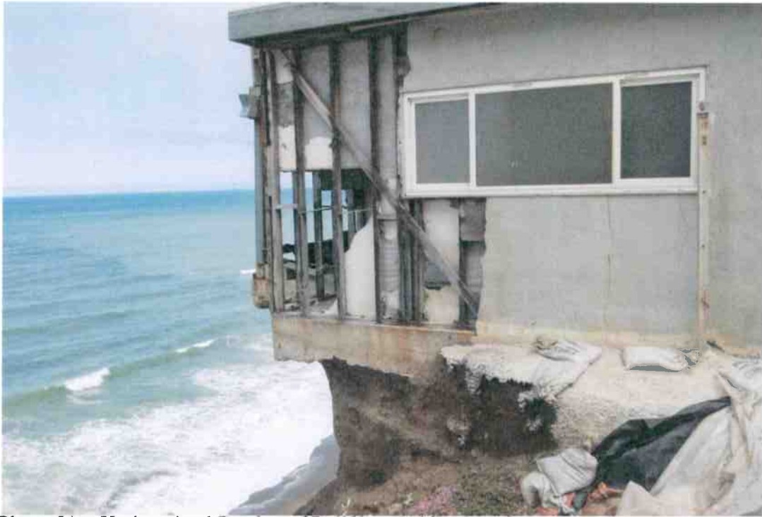
Photo 5A – Undermined Portion of Building, 320 Esplanade
