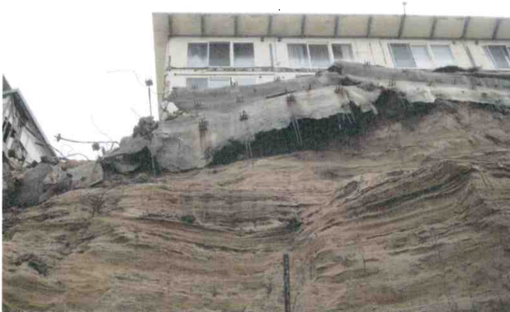
Photo 2A – Damaged and Partially Detached Shotcrete Facing, 330 Esplanade
