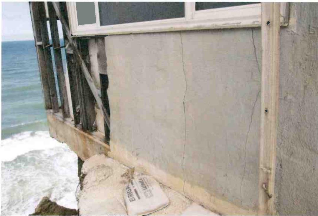
Photo 5B – Tensional Cracks, 320 Esplanade
